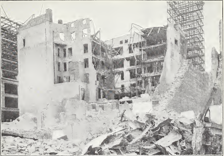
A. COLLAPSE OF BUILDING DUE TO BUCKLING OF COLUMNS, SPRING VALLEY WATER COMPANY'S BUILDING, SAN FRANCISCO.
